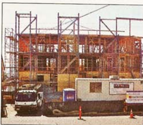
The Bankers Hill construction site, as of August 27. If you want to see the "bones" of a green project, this is for you.
